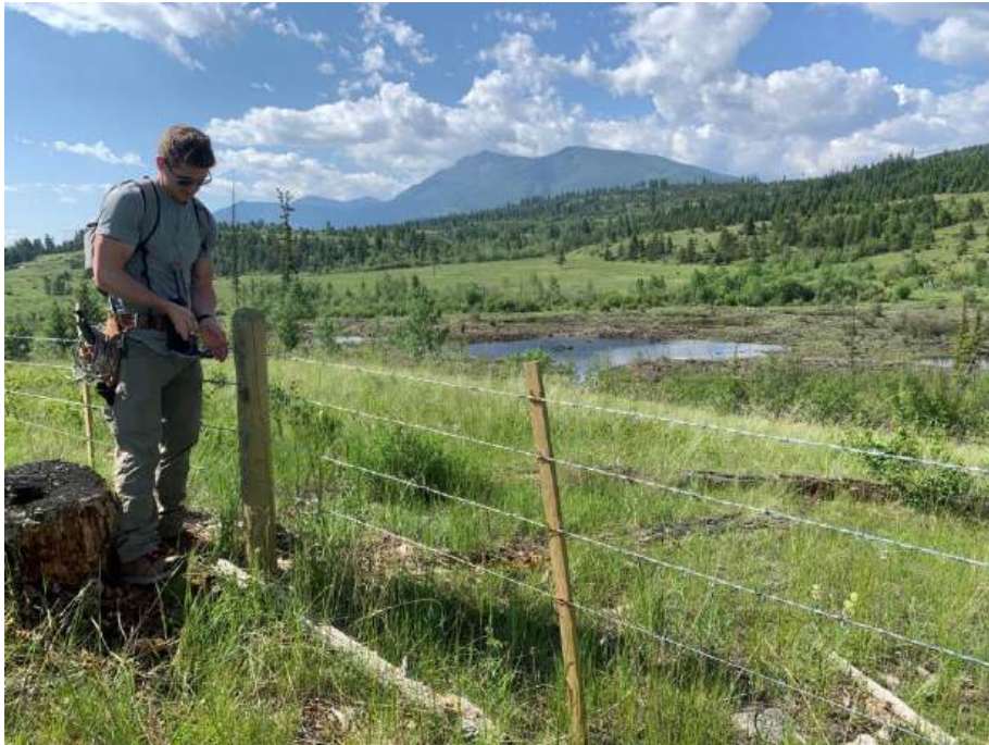
Figure 6: Replacing staples in a fenceline which protects the Sun Creek wetland restoration site from cattle and recreational trespass.
